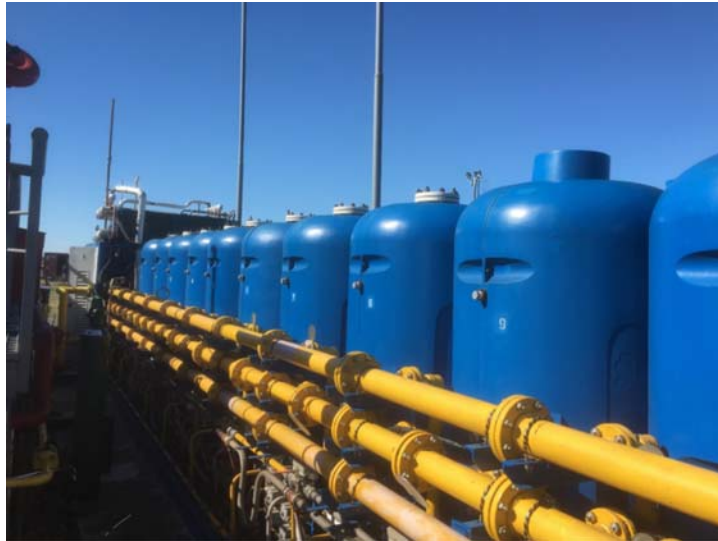
Galileo ZTPS - Raw Gas Treatment Plant
